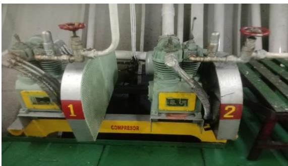
Gambar 1 Main Air Compressor
